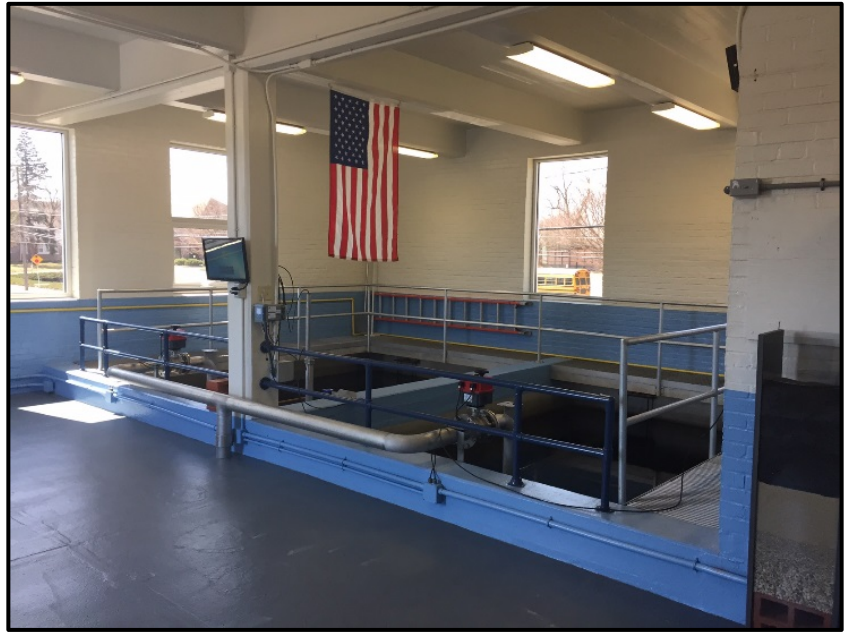
Figure: EAJA's Water Treatment Plant – Filter Room
