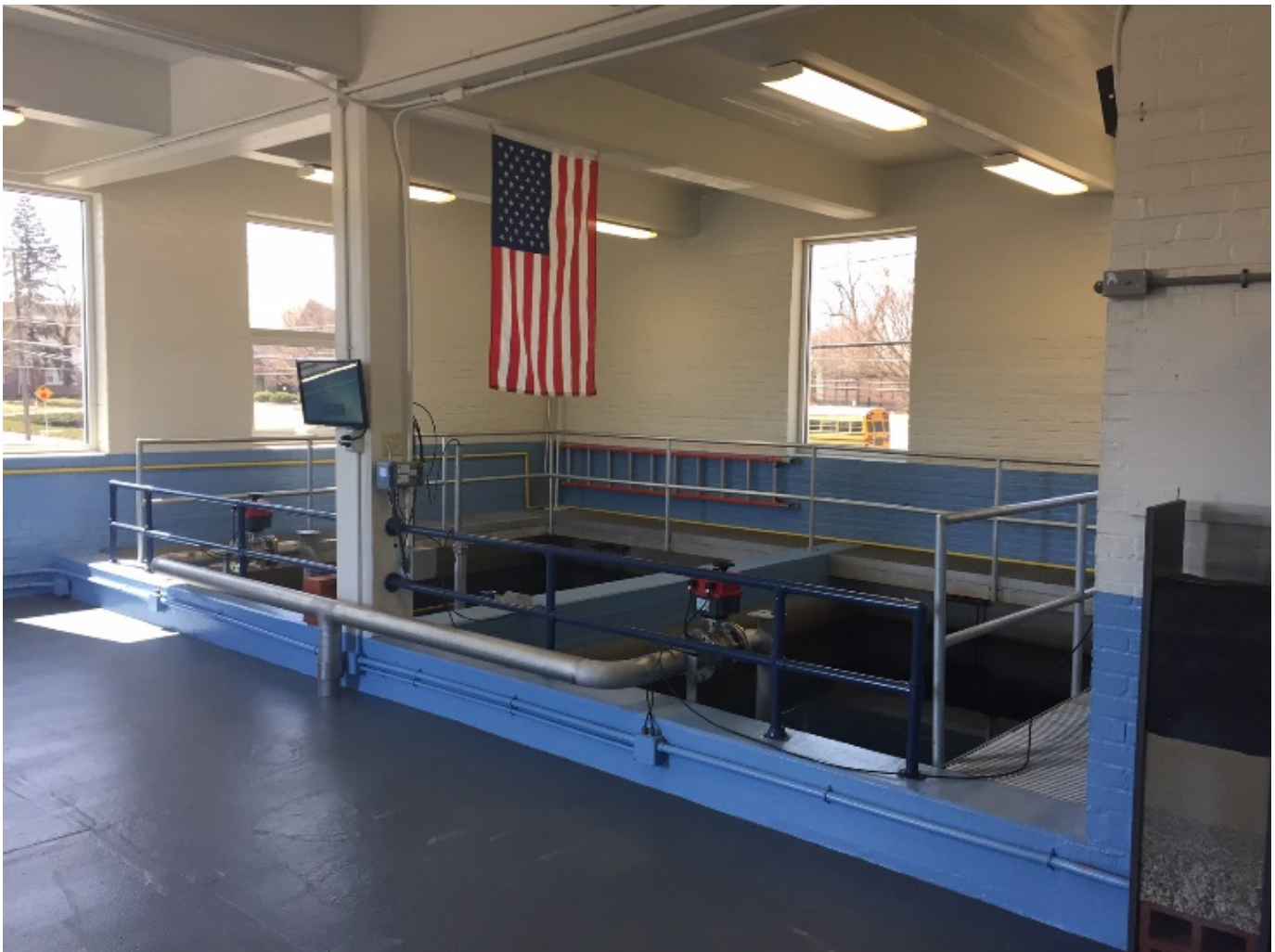
Water Treatment Plant – Filter Room
